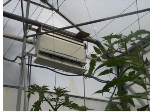
Figure 24. Picture of one heat exchanger with the condensate water collection device.
