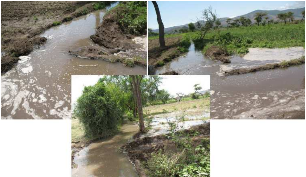
Figure 3.3a b, c over topping of the main canal
